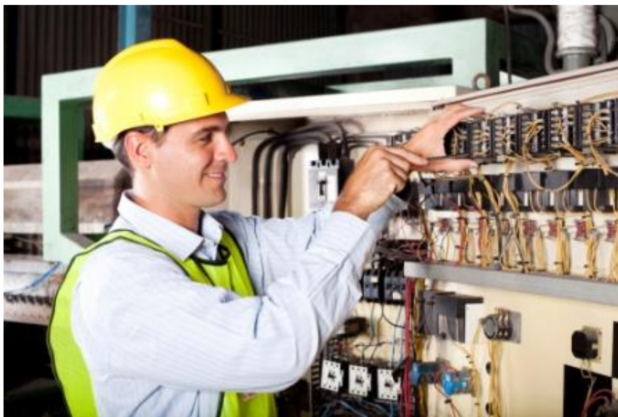
electrician reparing industrial machine
